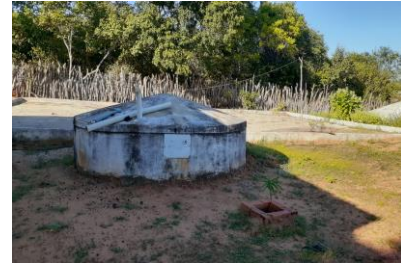
Fig.4: Cistern for rainwater collection and use.
