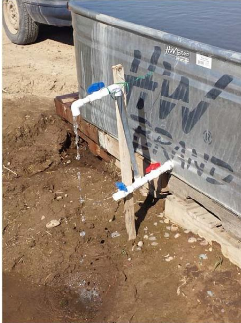
Figure 2 – Photograph showing the outlet of the simulated filtration pond constructed at Oregon State University Malheur Experiment Station, 2013.
